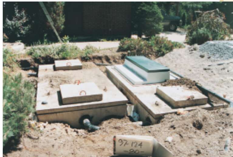
A typical aerobic treatment unit alongside the septic tank.
