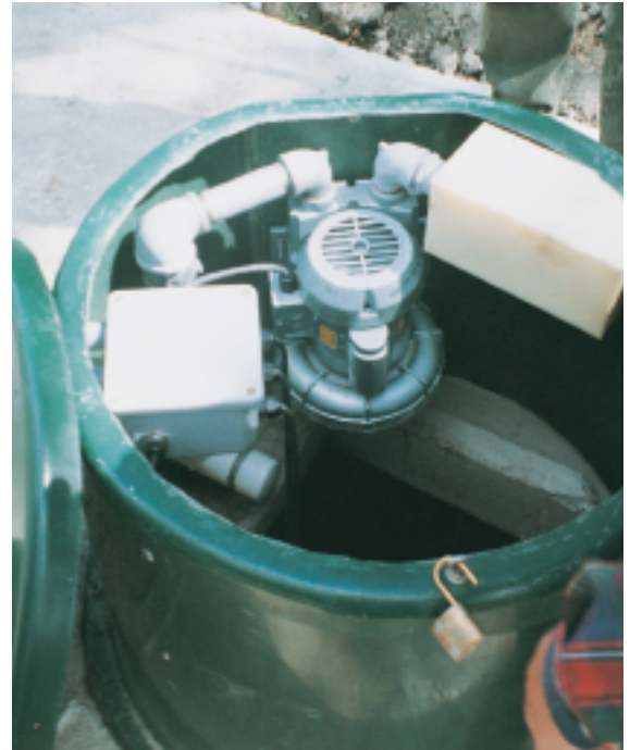
Aeration blower on an aerobic unit.
